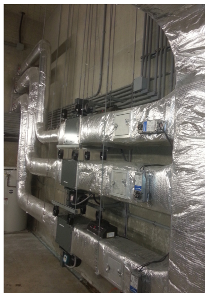
Hydroxyl generators were used in the HVAC system for chemical dosing rooms.
