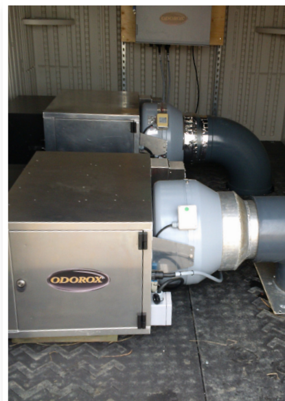
Hydroxyl generators installed on the upper vault.
